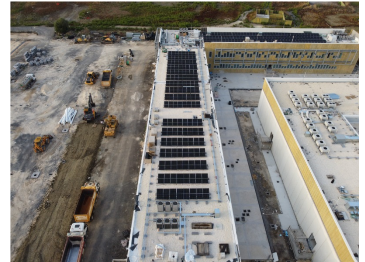
Solar panels on the roof – Design services NATO Main Operating Base in Sigonella, Italy
